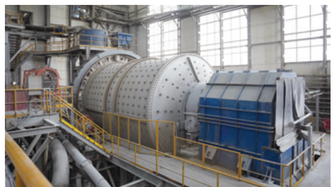
↑ Ball mill of the flotation plant.
